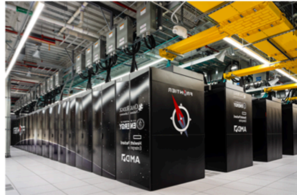
OLCF Frontier Cabinets deployed at ORNL
