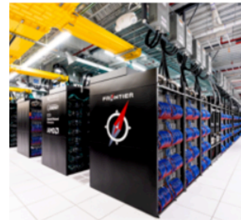
OLCF Frontier cabinets deployed at ORNL
